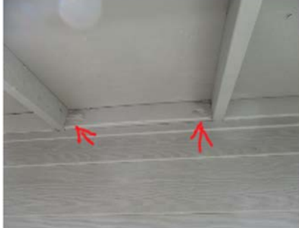
Bird Blocking Installed With Splintered Material
