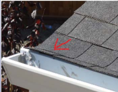
Roofing With Different Pitch Is Causing Composite Shingles To Rise When Gutters Installed
