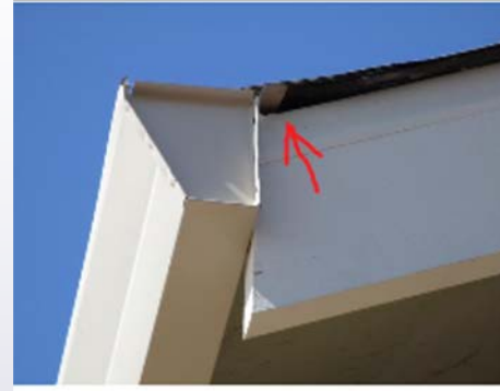
Side View Of Composite Roofing Raised Up Because Of Improper Gutter Install
