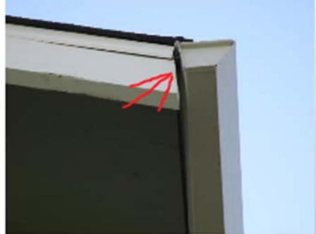
Roof Truss Ends Not Cut Square At Same Distance
