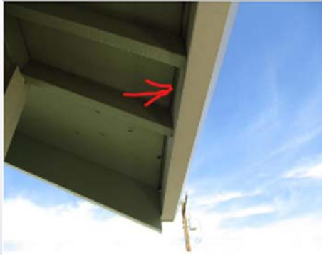
Roof Sheathing Is Not Cut Properly At End Of Roof Truss Ends
