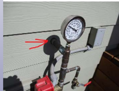
Plumbing Hole Penetration Needing To Be Sealed With Caulking
