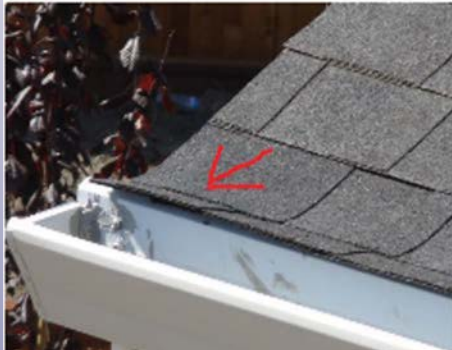
Roofing With Different Pitch Is Causing Composite Shingles To Rise When Gutters Installed
